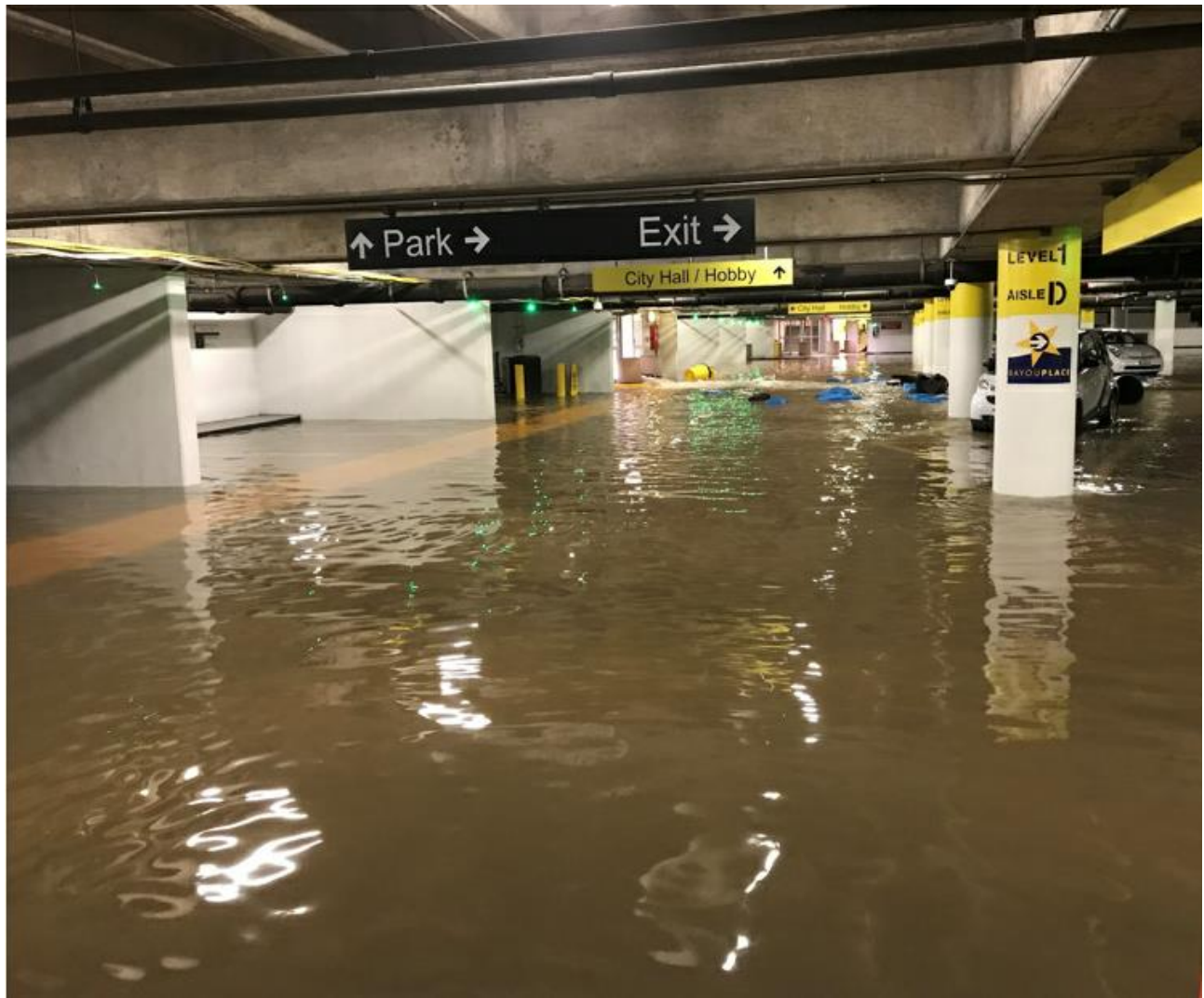
Figure 3. Flooding in Yellow Garage, First Level (August 27, 2017)
